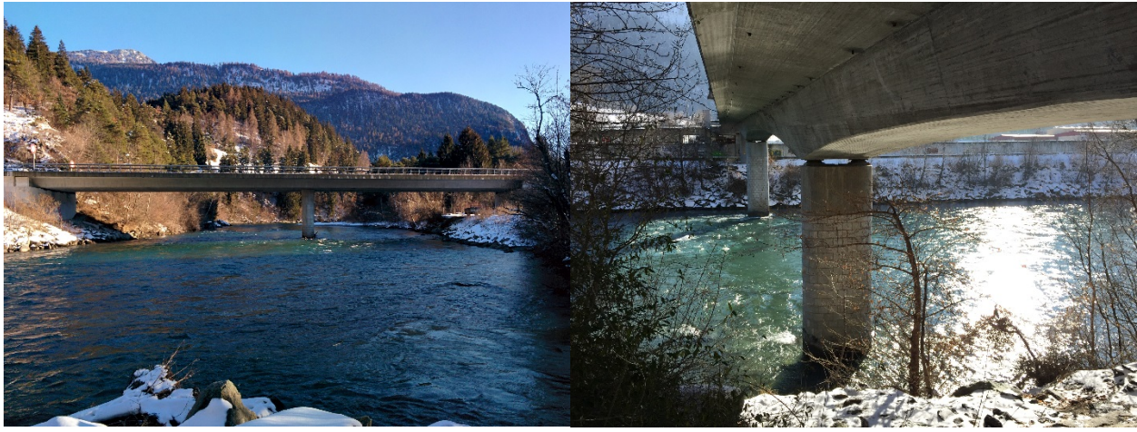
Figure 10 Examples of bridges in the area of study of (left) type A and (right) type B
